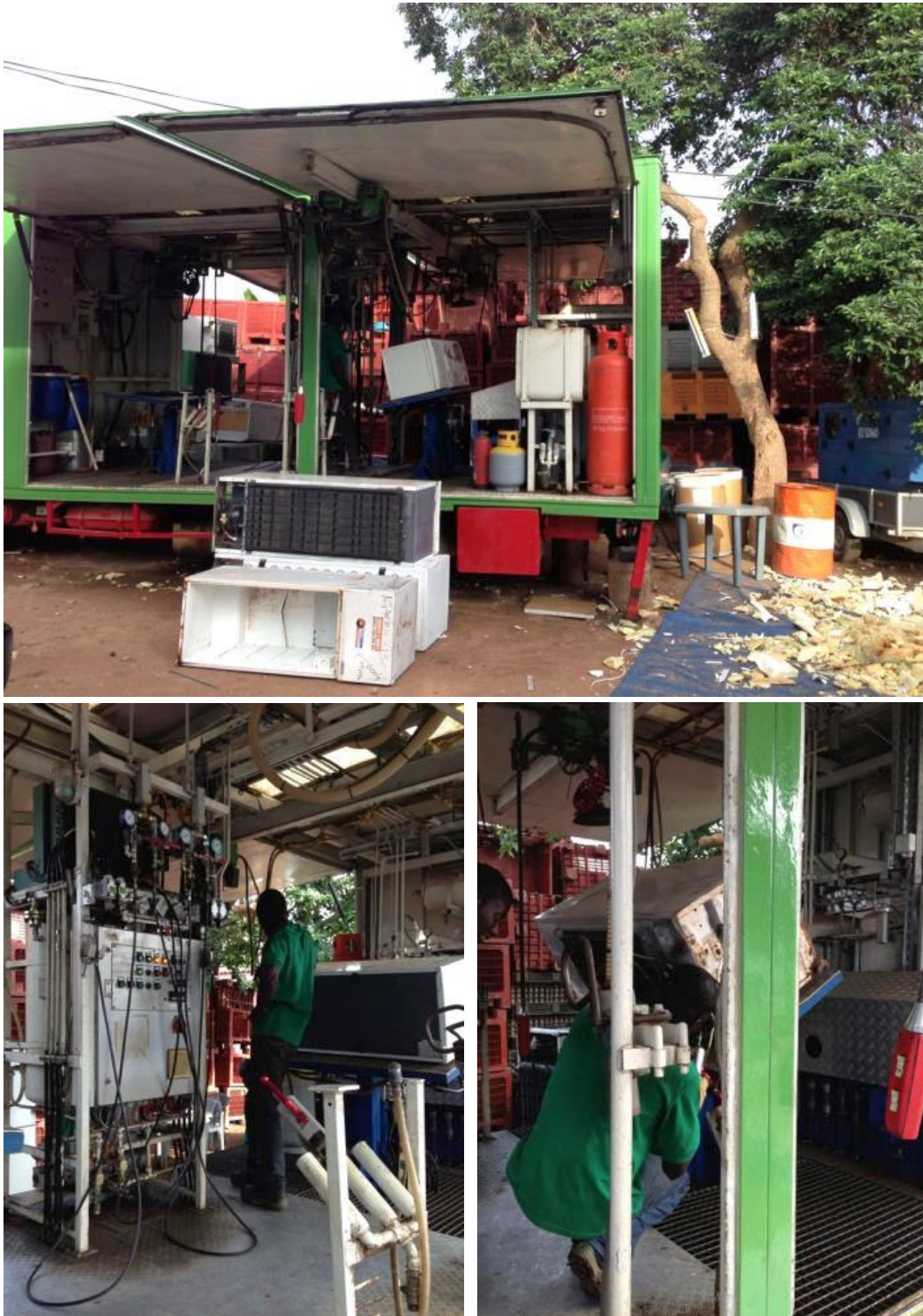
Figure 10: Formal refrigerator treatment in Ghana: mobile treatment plant for de-gassing of refrigerators (top); details on de-gassing operations (bottom left) on a refrigerator.
